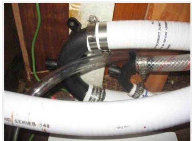
NEW Holding Tank
