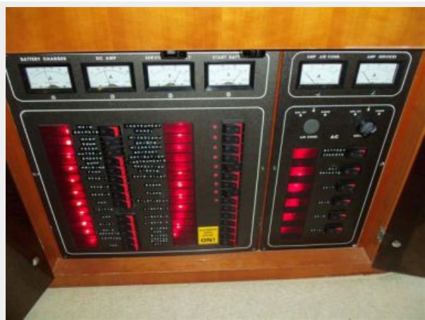
Pilothouse Electrical Panel
