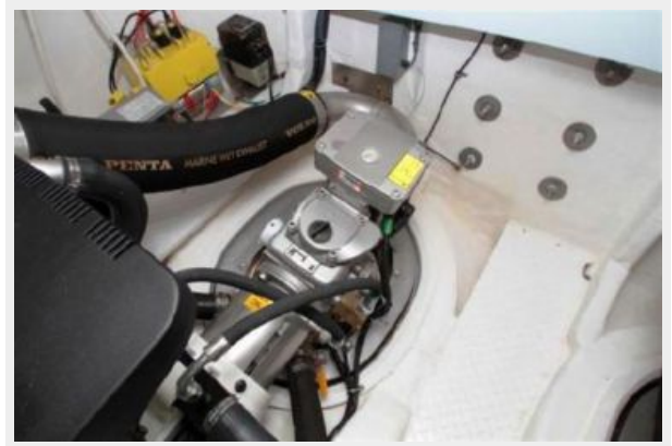
Expansive Engine Room
