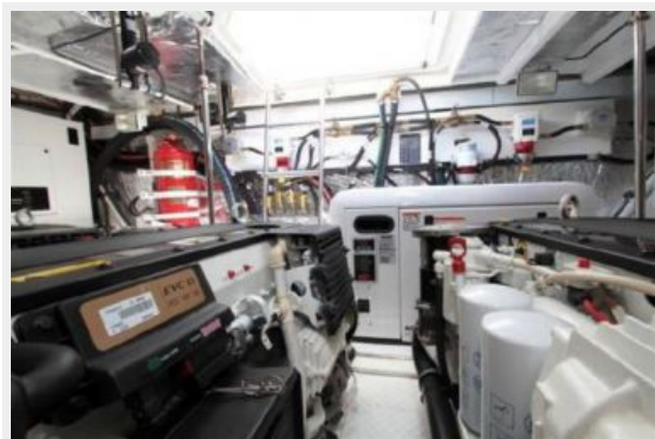
Expansive Engine Room
