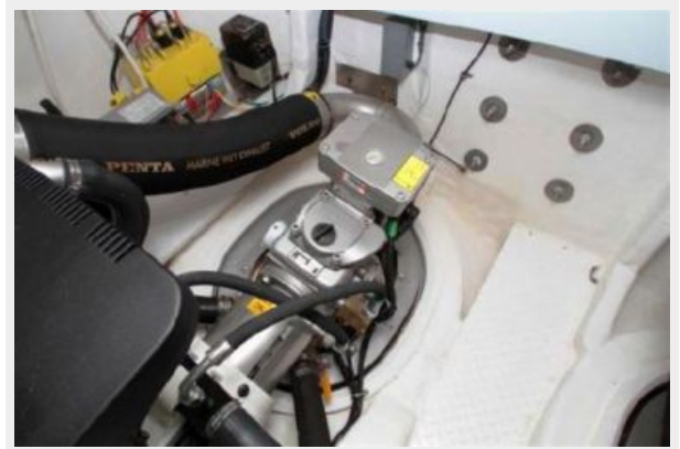
Expansive Engine Room
