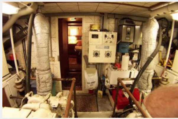
Engine Room Aft
