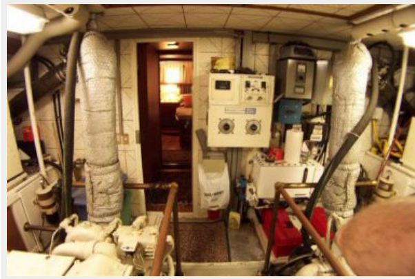
Engine Room Aft
