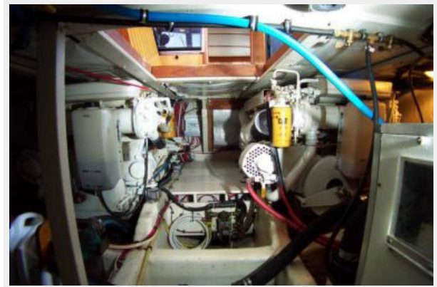
Clean Engine Room
