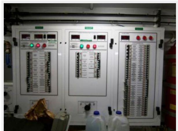
Engine Room Equipment
