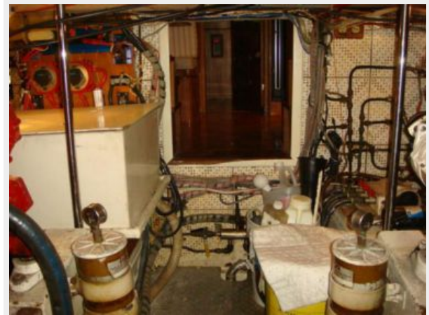
43' Tradewinds Engine Room Forward
