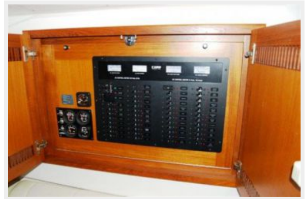
Electrical Distribution Panel
