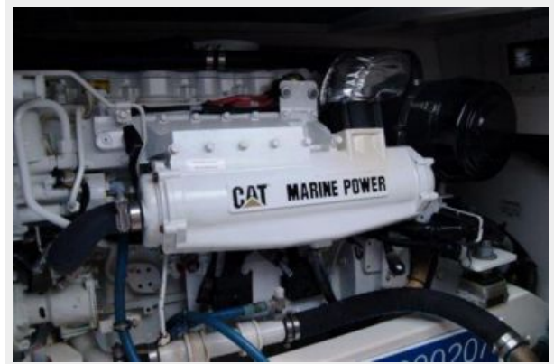
Starboard Main Engine
