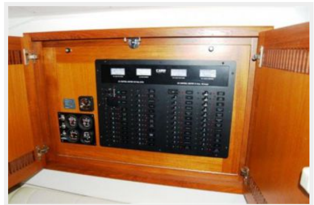
Electrical Distribution Panel
