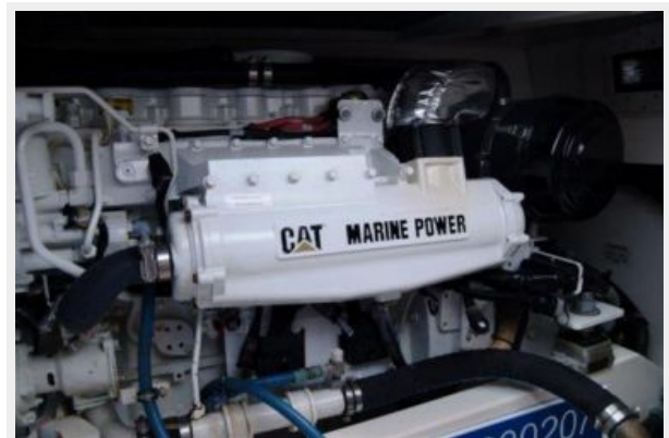
Starboard Main Engine
