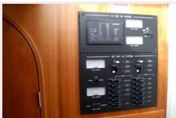
Electrical Distribution Panel
