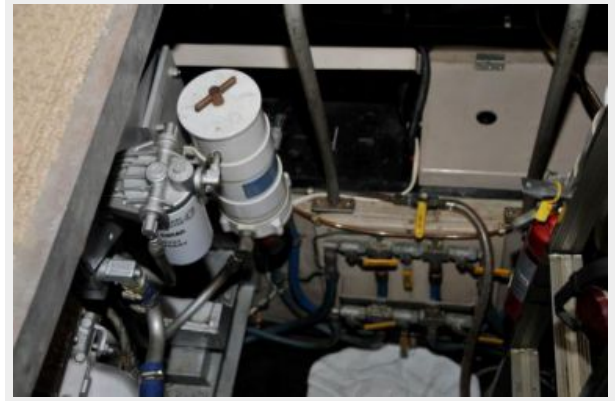
Engine Room Details
