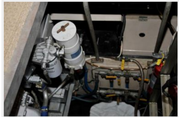
Engine Room Details
