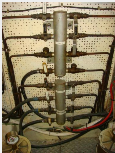
49' DeFever Fuel Manifold
