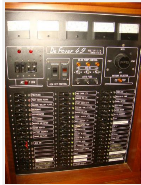
49' DeFever Electrical Panel
