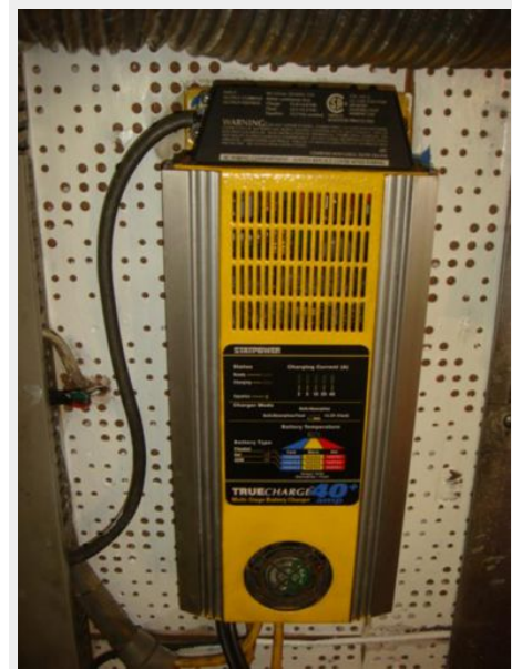
49' DeFever Battery Charger
