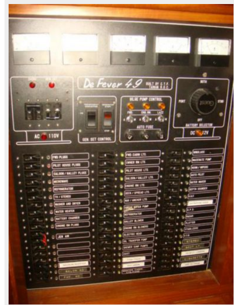
49' DeFever Electrical Panel
