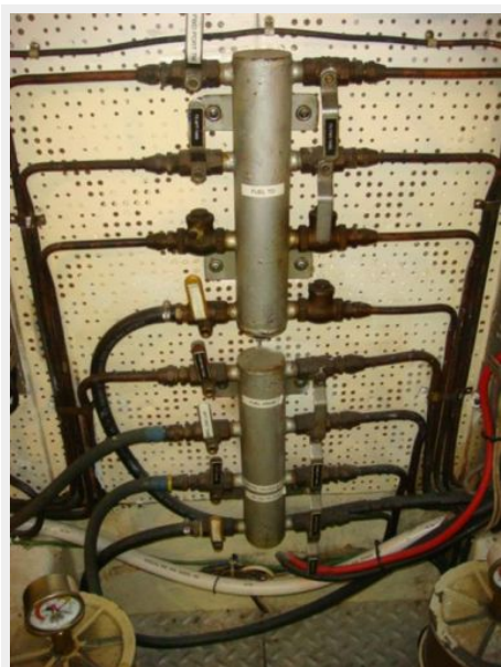
49' DeFever Fuel Manifold
