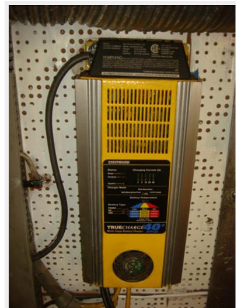
49' DeFever Battery Charger
