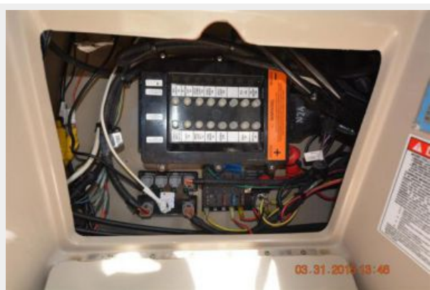
Wiring below helm
