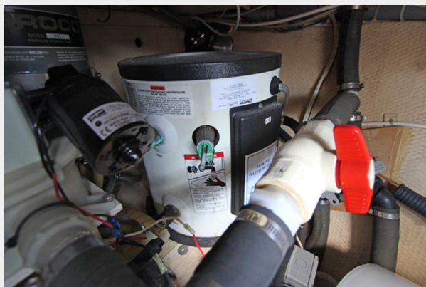
Hot Water Heater
