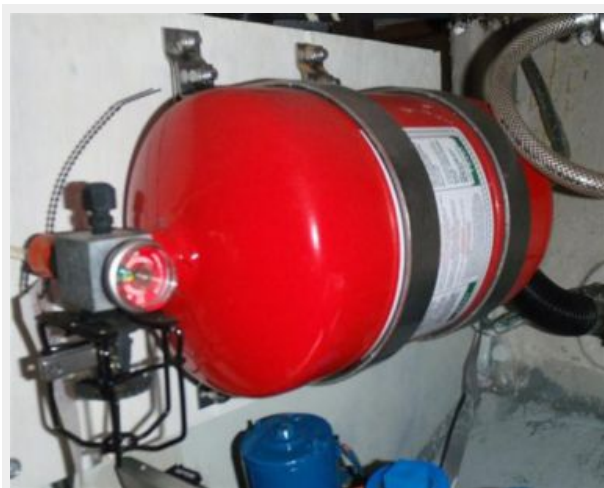
Fire Suppression System
