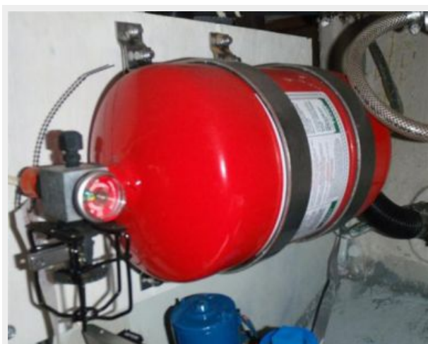
Fire Suppression System
