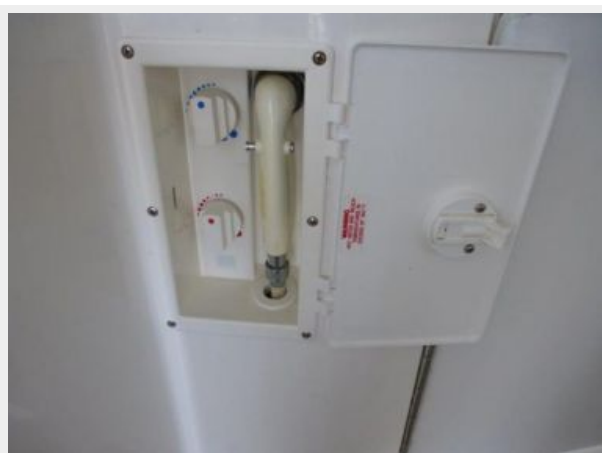
Aft Deck Hot/Cold Shower
