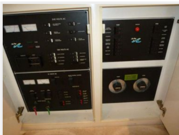
Main Distribution Panel
