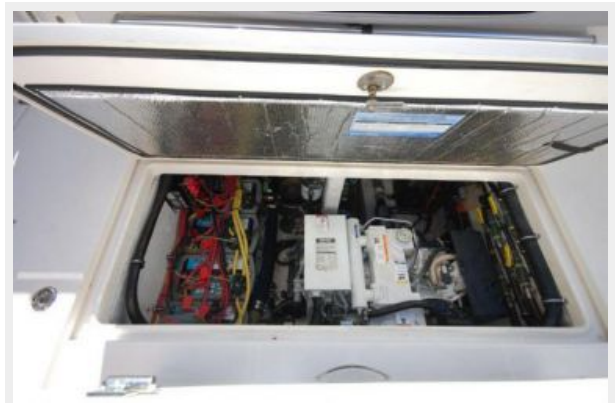
Generator and Batteries
