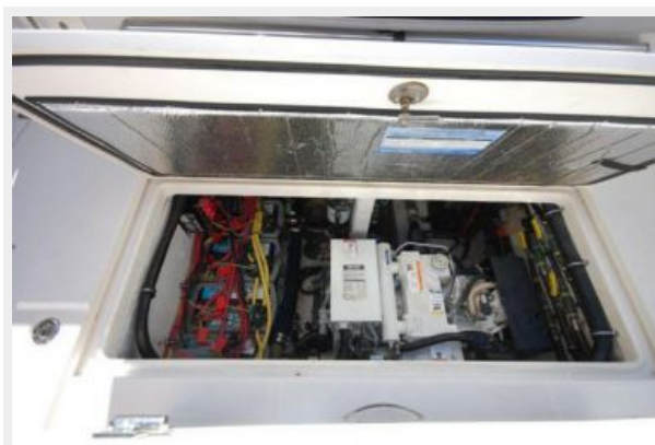
Generator and Batteries
