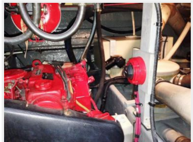
Generator in the Engine room
