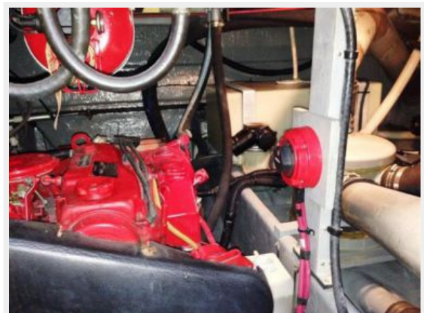
Generator in the Engine room
