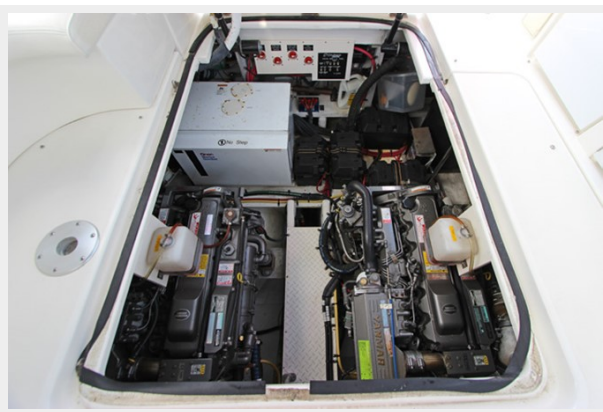
Engine Compartment with great access to engines, genset, all systems
