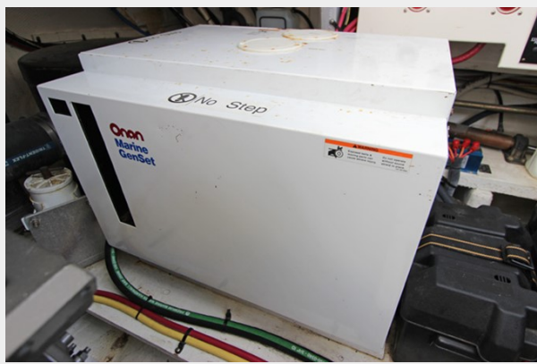
Onan 6.5KW Generator w/323 hours & sound shield
