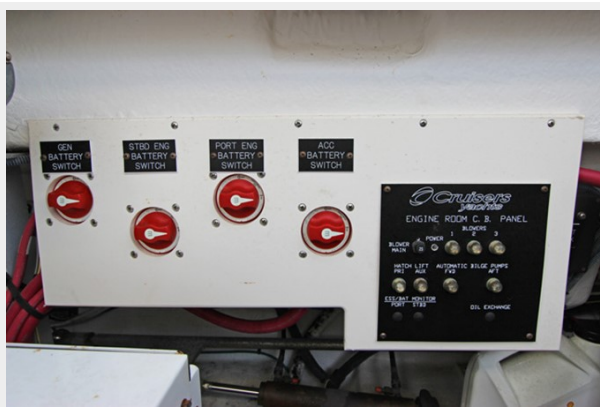
Engine Room Electric Panel w/switches for Generator/Engine/House Batteries
