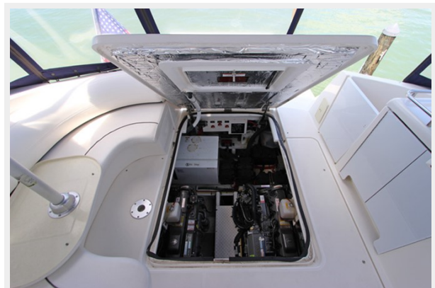
Electric Engine Compartment Hatch in Cockpit Sole
