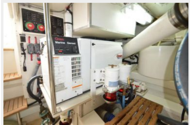
'07 Eastbay 47 FB, Generator
