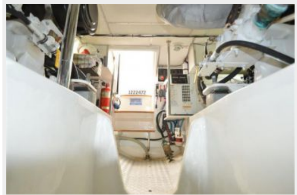
'07 Eastbay 47 FB, Looking Aft in Engine Room
