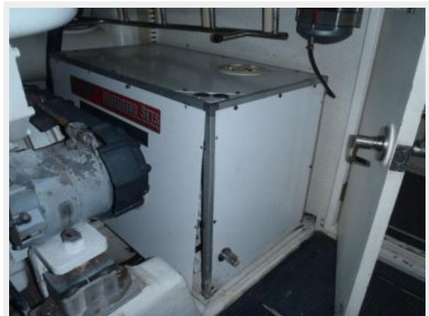
Generator in sound shield
