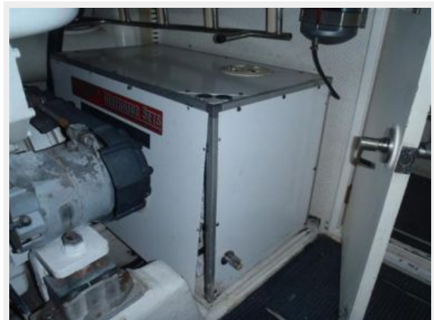
Generator in sound shield
