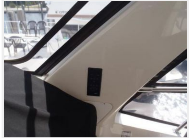
Bridge A/C control
