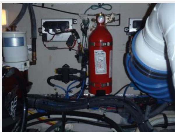
Fire suppression system
