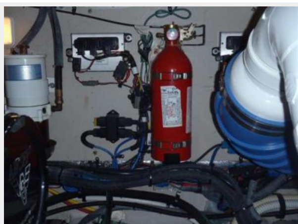
Fire suppression system
