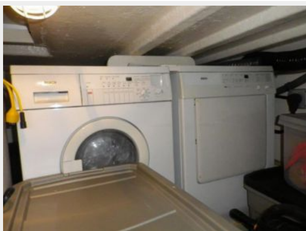
Laundry in Engine Room
