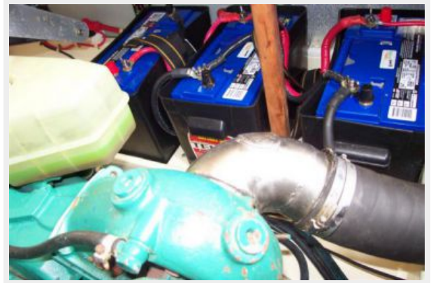
AGM Batteries - New 11/2013
