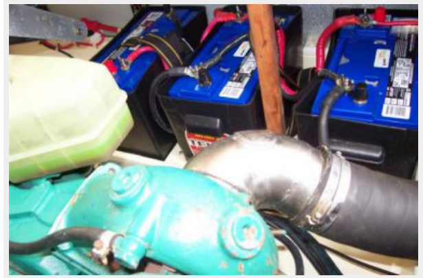
AGM Batteries - New 11/2013
