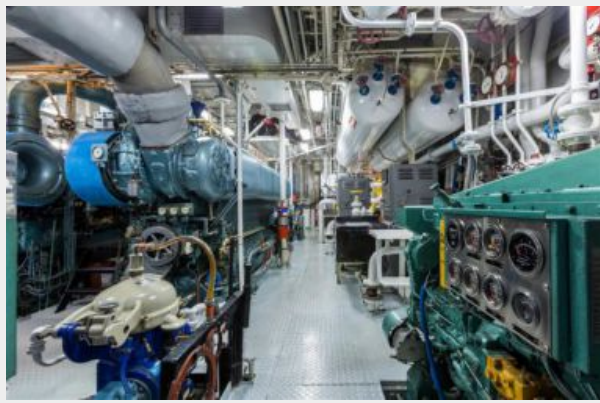
22_180712_ITASCA_Engine room_Hi-1309- credit Quin BISSET
