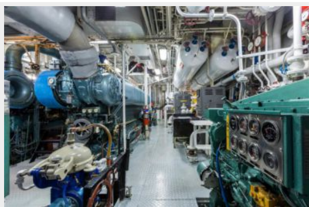
22_180712_ITASCA_Engine room_Hi-1309- credit Quin BISSET
