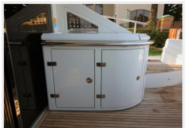
Aft Deck Electrical Panel
