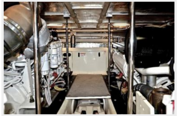
Engine Room Forward
