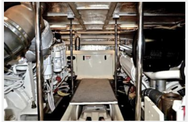
Engine Room Forward
