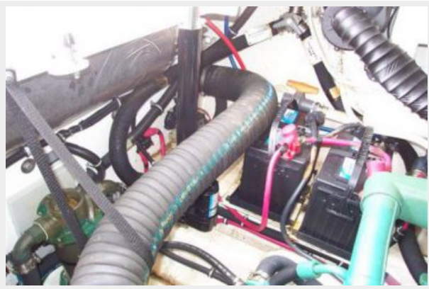
NEW Batteries (4) Group 27
