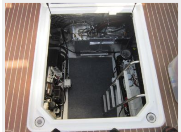
Engine Room Access
