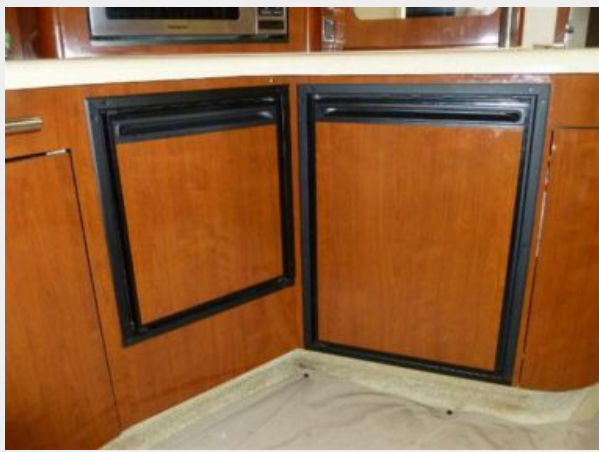
Galley Refrigerator and Freezer
