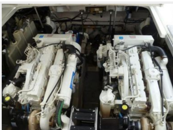
Engine Room overview
