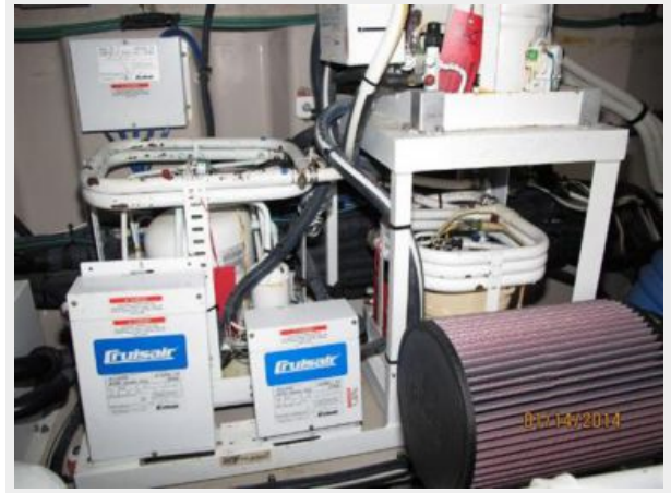
Starboard Side AC Units
