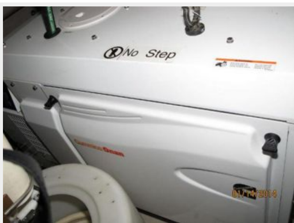
Generator Quiet Box
