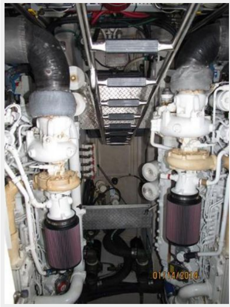
Engine Room Entry
