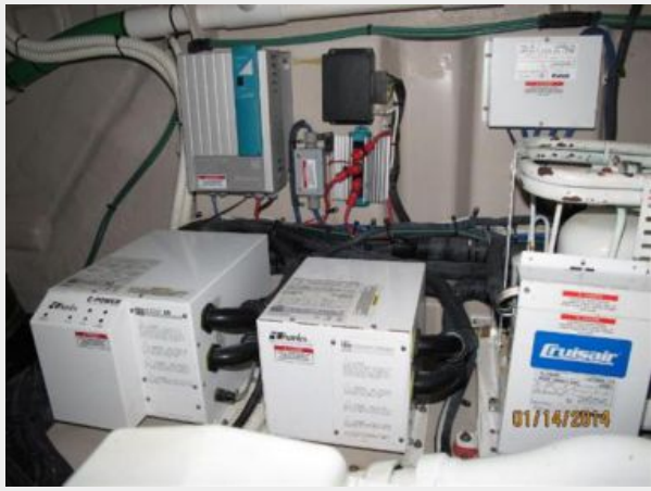
Engine Room to Starboard
