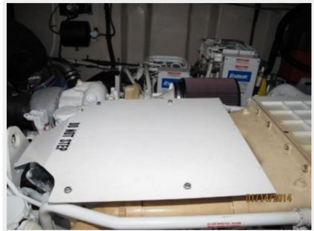
Engine Room to Port
