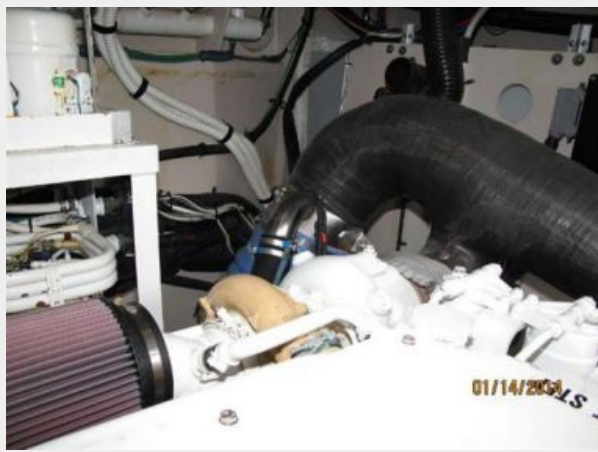
Engine Room to Starboard Forward
