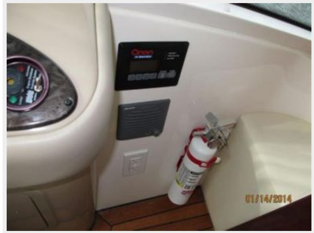
Remote Generator Panel
