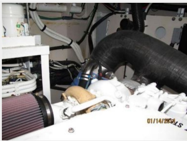
Engine Room to Starboard Forward
