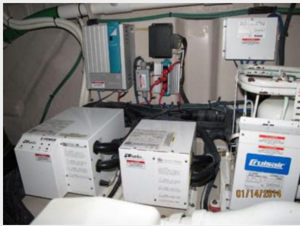
Engine Room to Starboard
