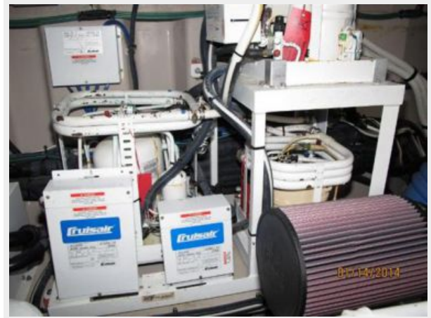
Starboard Side AC Units
