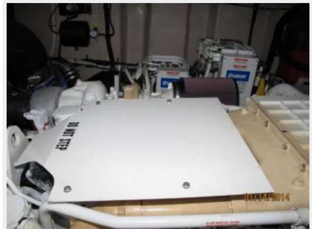
Engine Room to Port
