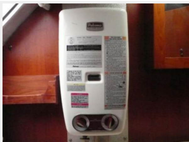
Hot water heater
