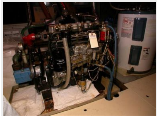
Bow Thruster Diesel/Hydraulic Power - Forward machine room located under galley
