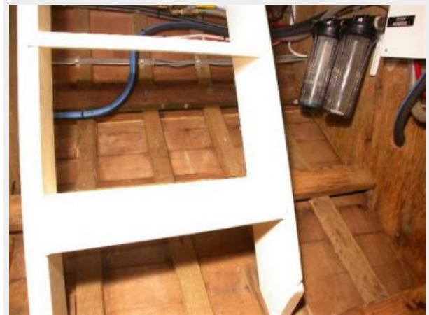
Stair to forward machine room - Forward machine room located under galley
