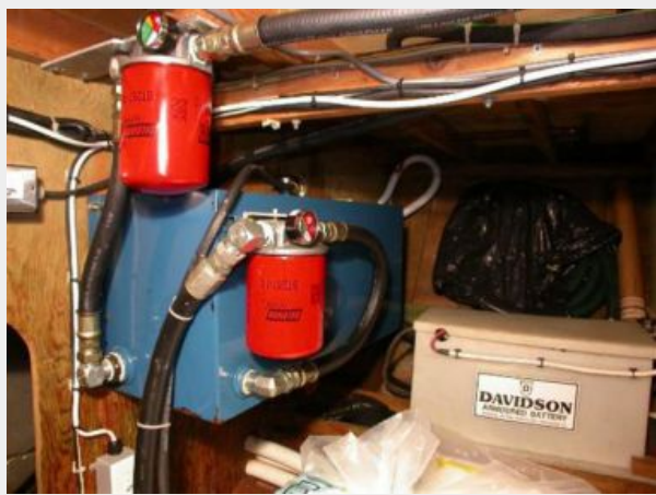
Bow Thruster Hydraulics - Forward machine room located under galley
