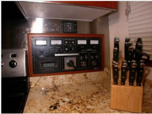
Galley Elect Load Center
